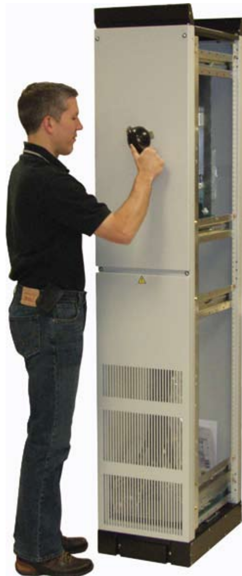
Incomer with disconnect shown with side panel removed for illustration purposes.
