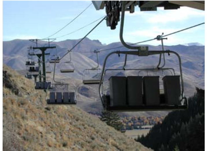
Testing a retrofit drive installation
